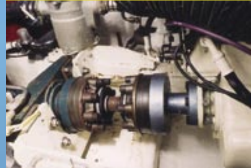
Aquadrives installed with 400hp engines on a 15m motor yacht.
